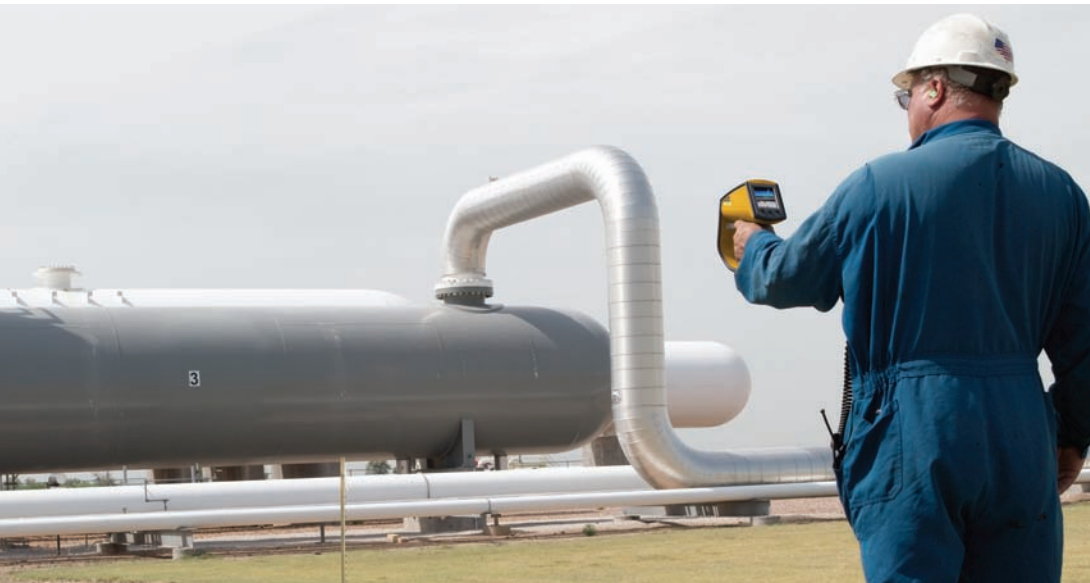
Figure 1. Checking tank levels at a natural gas processing facility.
